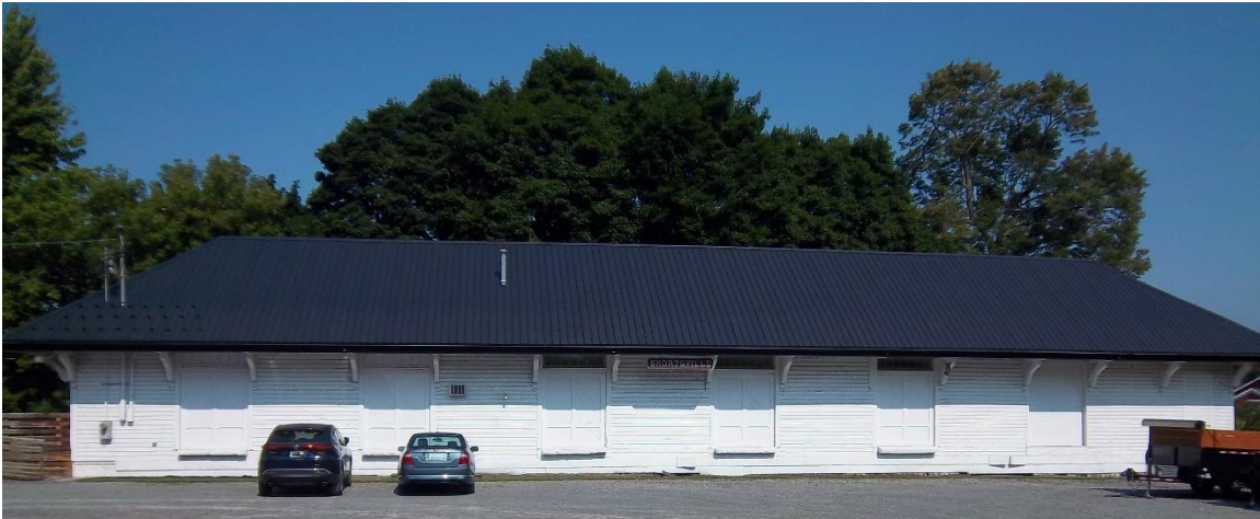
View of New Roof on East Side of LVRRHS Station Museum (Ken May Photograph)
